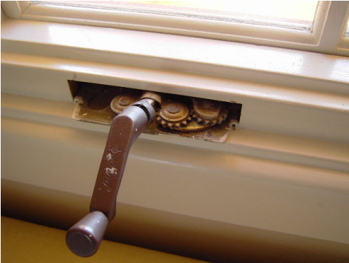
Photo of missing and inoperable hardware.
