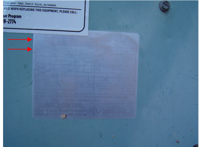
Please note photo of label. The model and serial numbers are faded beyond recognition.
