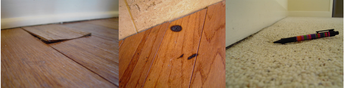
Peeling floor right of fireplace.
